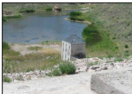
The drain in the Little Puerco Wash is typically dry and visible during most of the year.
