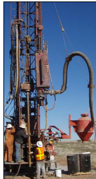
The Bar-Cad multilevel groundwater monitoring system allows water samples to be taken from different depths.
