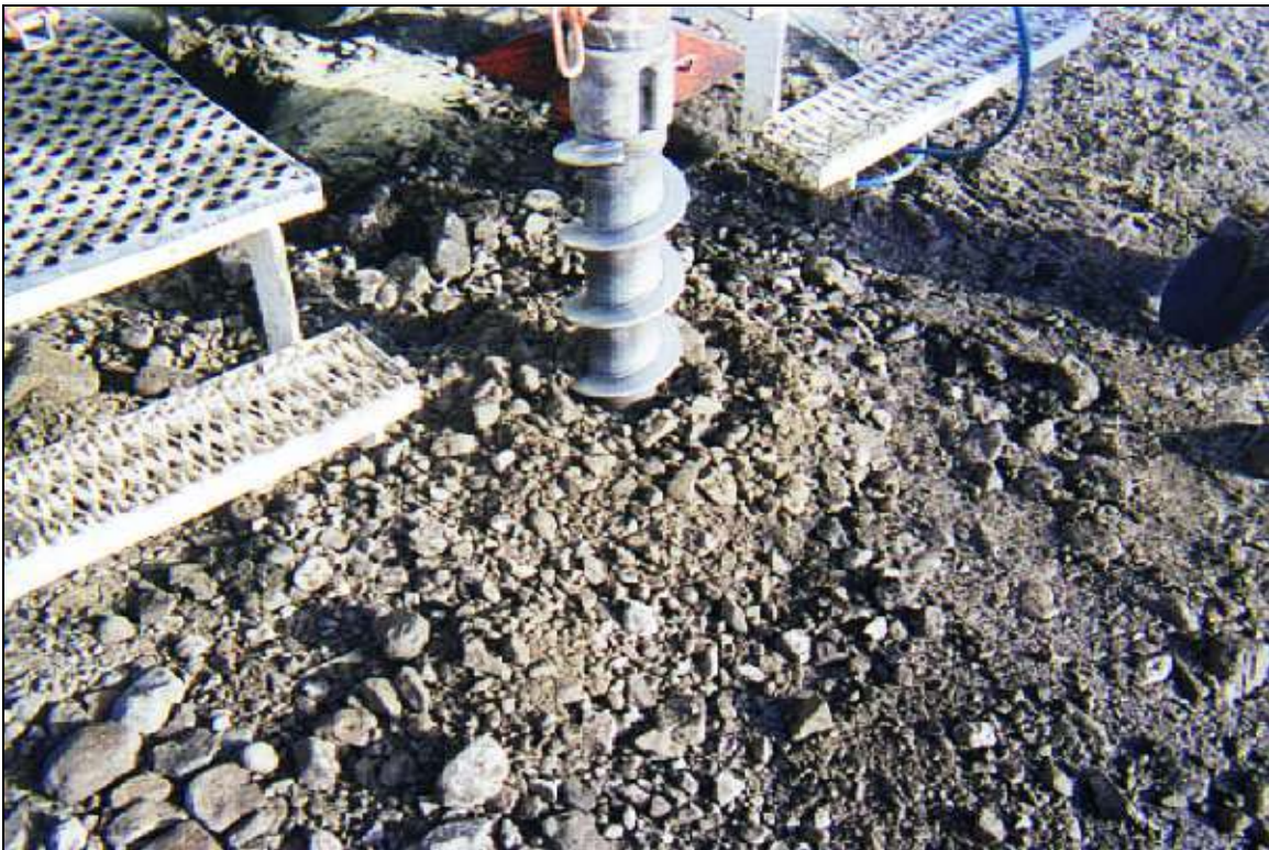
Photograph 8: Damp Cuttings at MW19 Indicating Groundwater
