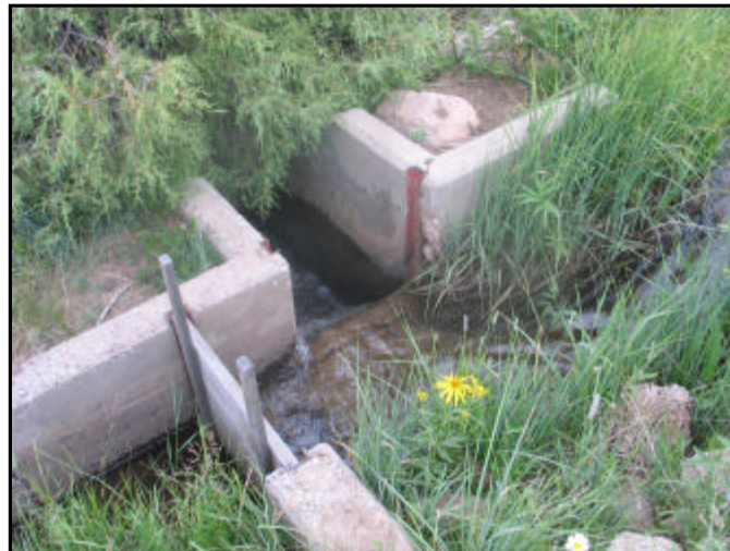
Figure 1-3. Branching to primary lateral – lateral flows toward upper left of photo.
