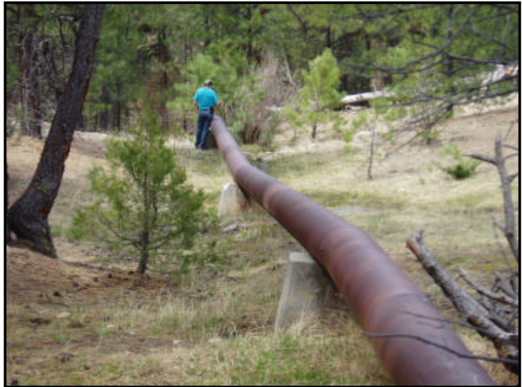
Figure 1-5. Previously installed inverted siphon
