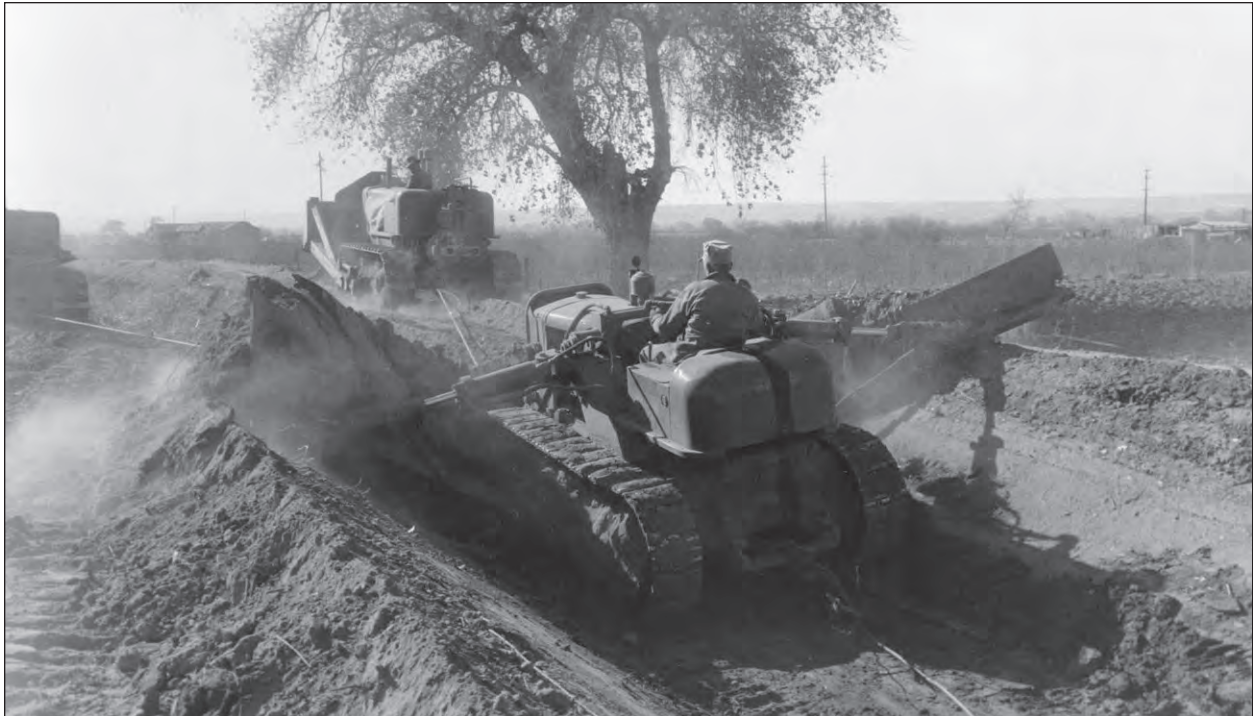
Figure 30. Specialized equipment (“ditcher with spoil wings”) designed for renovating MRGCD structures at Los Chavez Acequia, 1956 (compare with Figure 17). Source: USBR.
