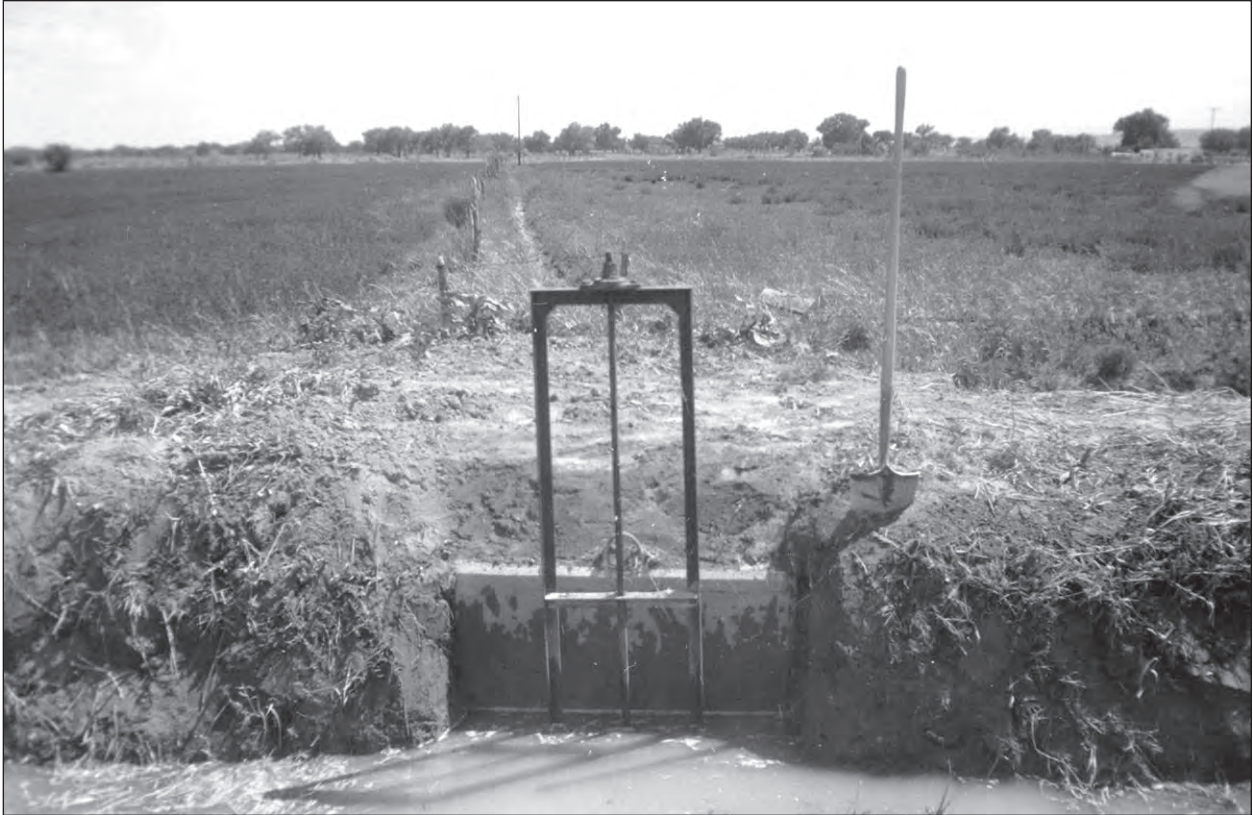
Figure 62. Metal turnout and precast concrete headwall installed on Old Jarales Acequia, 1957. Source: USBR.
