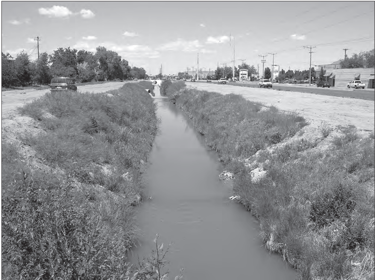
Figure 68. Alameda Interior Drain, looking north along Second St., 2007. Note water coming out of culvert from adjacent land formerly used for farm fields, but now built up with suburban housing. Compare with Figure 54. Source: VCHP.
