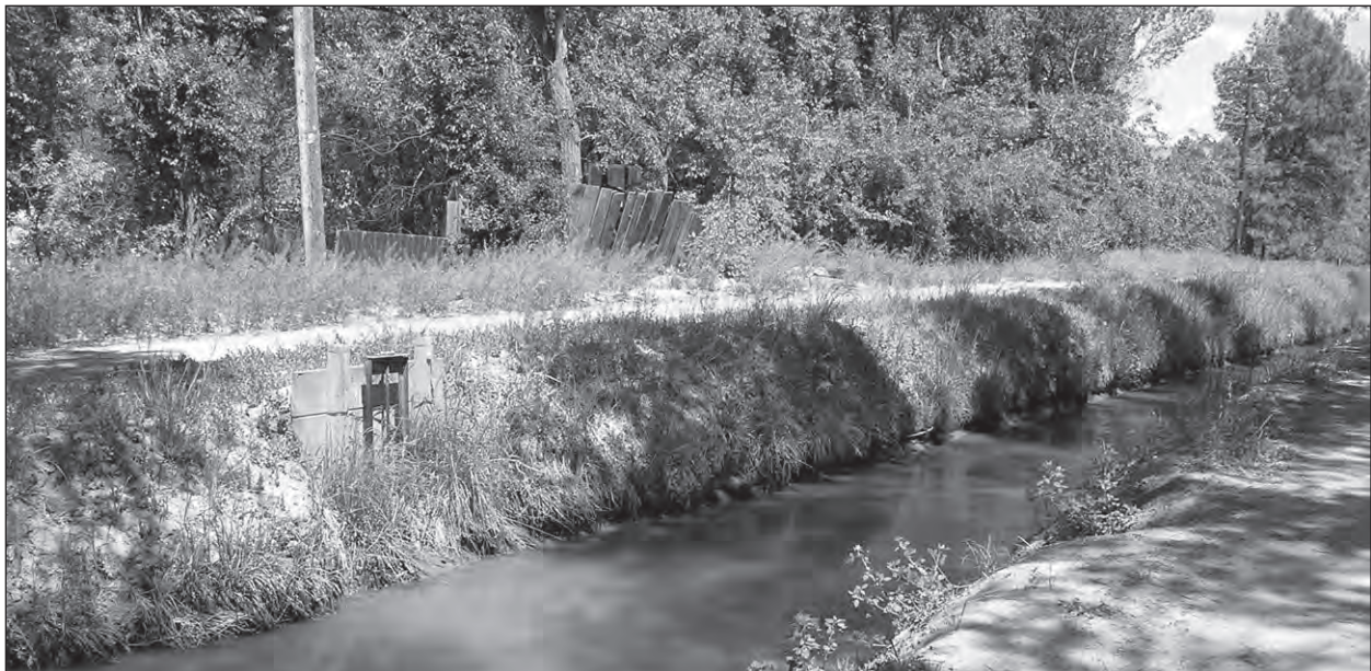
Figure 57. Acequia turnouts located along the Gallegos Lateral in the North Valley, 2007. Source: VCHP.
