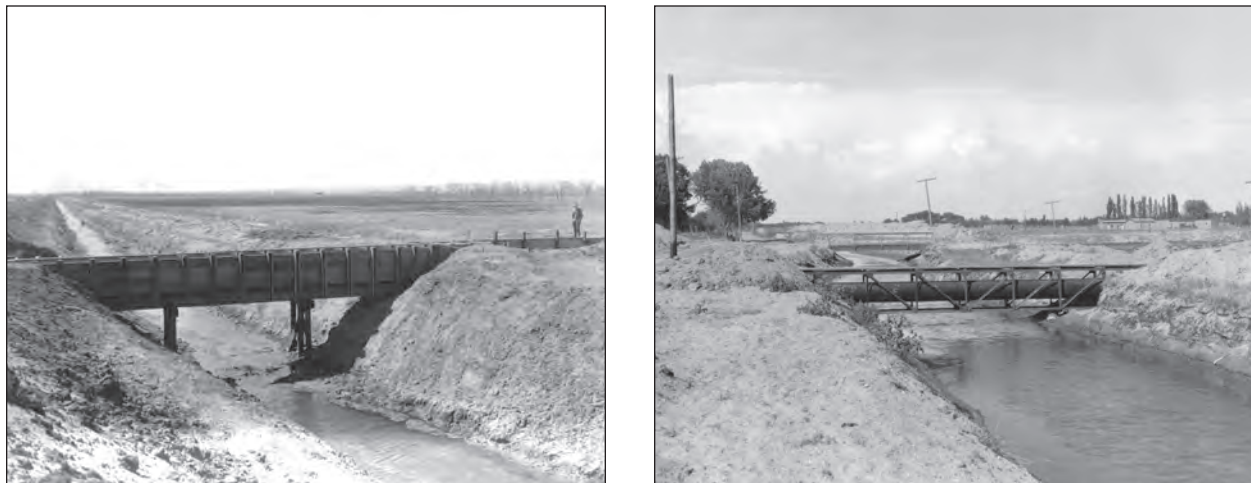
Figure 65. Gallegos irrigation flume crossing the Alameda Interior Drain, 1930; Covered flume carrying irrigation water over the Alameda Interior Drain near Old Town, 1930. Source: MRGCD.
