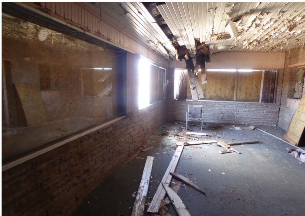
Figure 14. Interior damage including collapsed ceiling.
