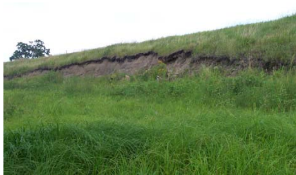
Figure 2.17 UNACCEPTABLE earthen embankment failure. (MN)
