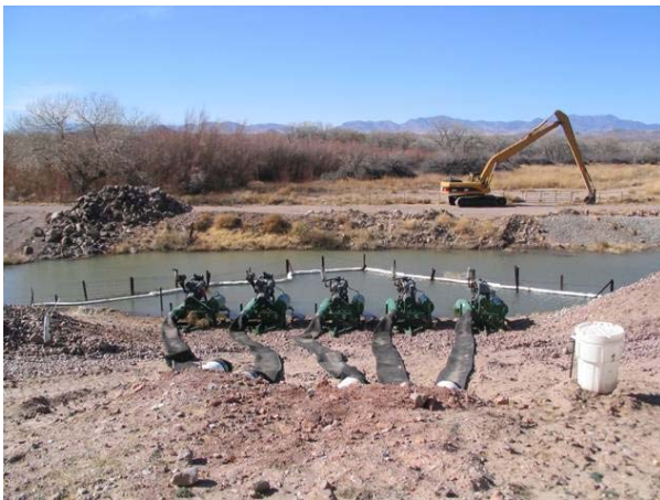
Figure 2.16. Low Flow Conveyance Channel Pumps
