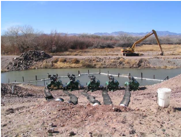
Figure 2.15. Low Flow Conveyance Channel Pumps
