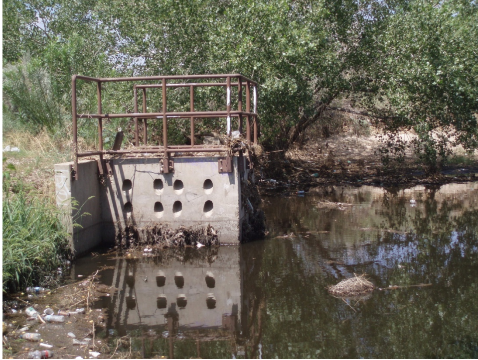
P3: Looking north at trash removal pond's vertical concrete intake. Note abundant trash/debris, clogged ports
