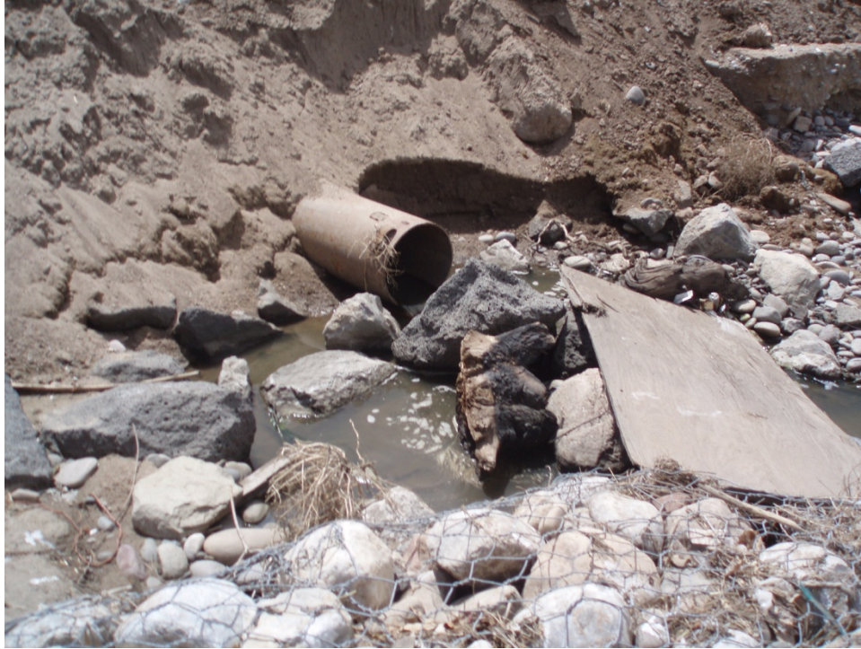
P14: Looking at discharge pipe from NDC settling basin into embayment. Photo location not shown on photo log.
