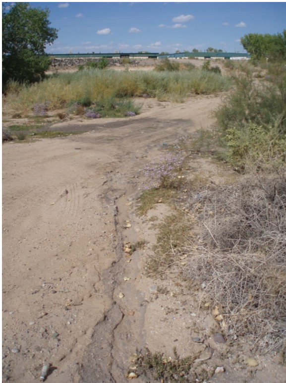
P8: Looking northwest, on the southwest corner of debris bins. Note discolored drainage from bins. Drainage crosses earthen access road in foreground and is conveyed into Pino drainage area on left.
