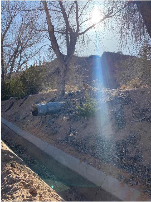
7. Looking East up channel of the Acequia De Sombrillo. Existing arroyo drain culvert seen at the top of the embankment.
