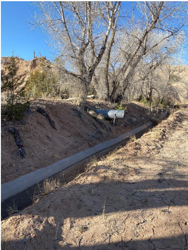
6. Looking West down channel of the Acequia De Sombrillo. Existing arroyo drain culvert seen at the top of the embankment.
