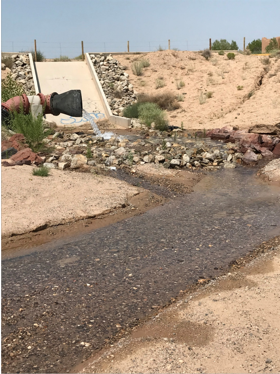
Black Arroyo Location 3 Site Visit 8/21/2020
