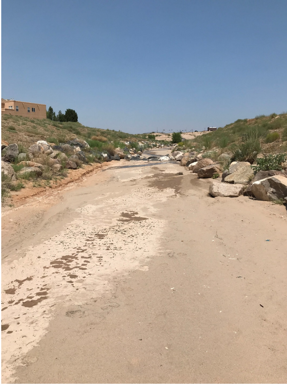
Black Arroyo Location 3 Site Visit 8/21/2020
