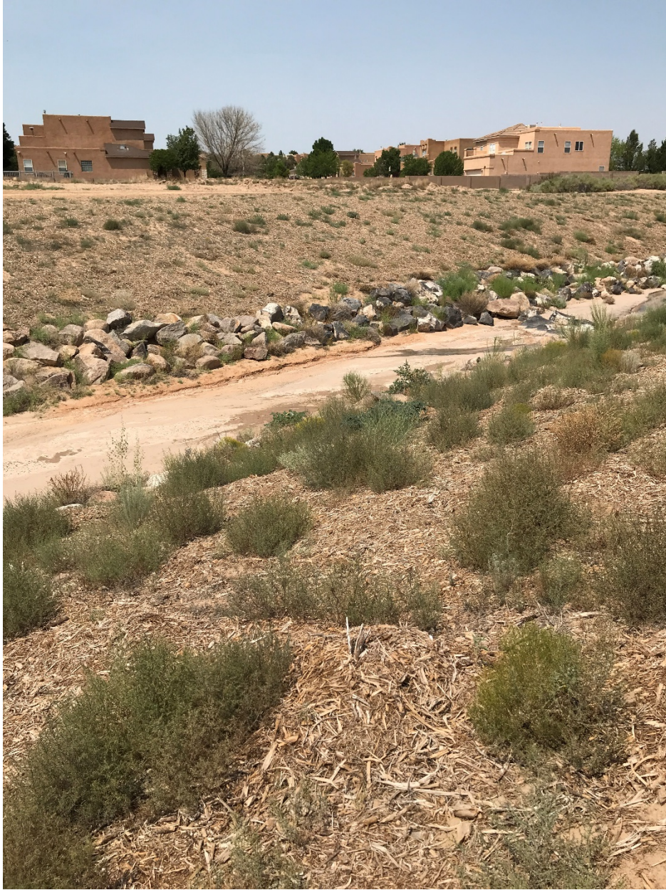
Black Arroyo Location 3 Site Visit 8/21/2020
