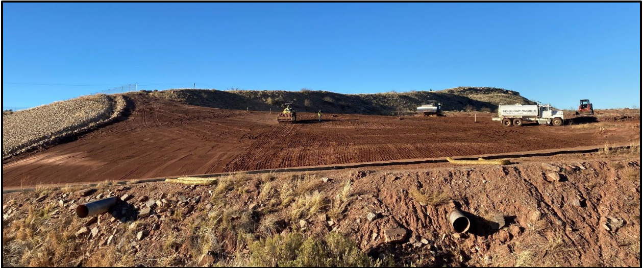
Photo 6-3 Erosion Mitigation at Conchas Lake
